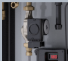
High Flow Recovery Pump
